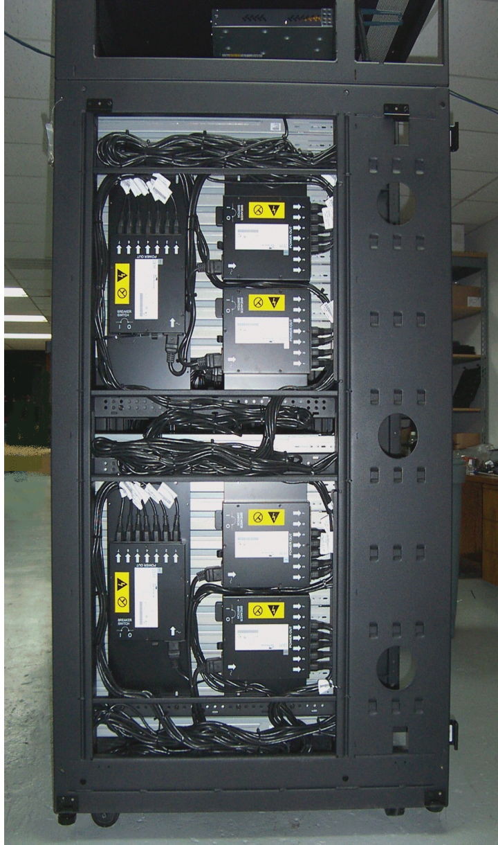
Figure 3-4 Power distribution units
