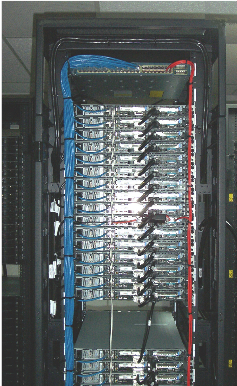
Figure 3-5 Cluster Ethernet, MPN, and C2T cabling
